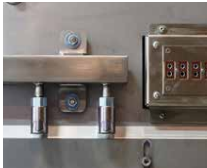
Connections for vacuum pump and batch thermocouples
